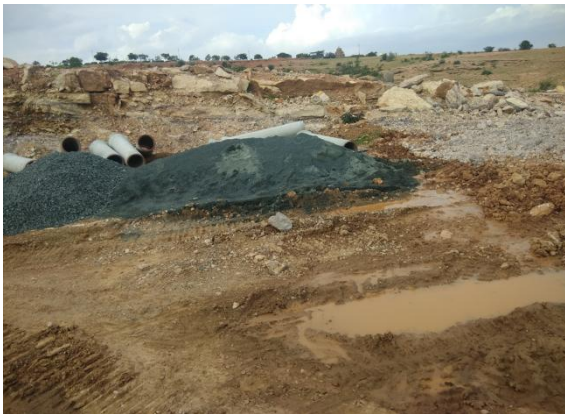
Bulk Services – pipes for drain water
