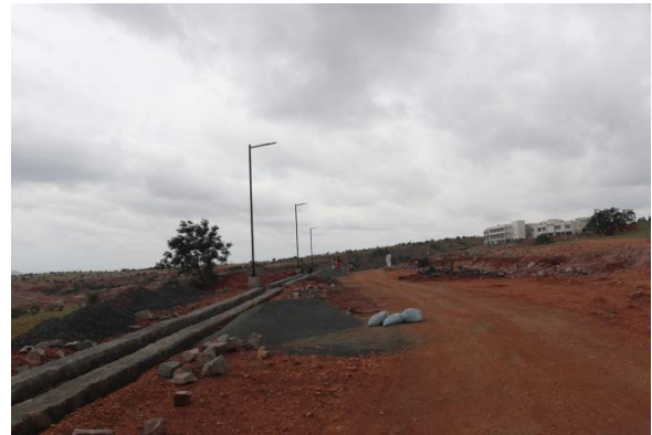
Bulk Services – street lights
